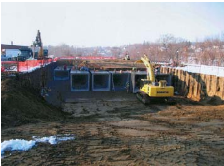
Category A. City of Lewiston Water St. CSO Storage Facility
